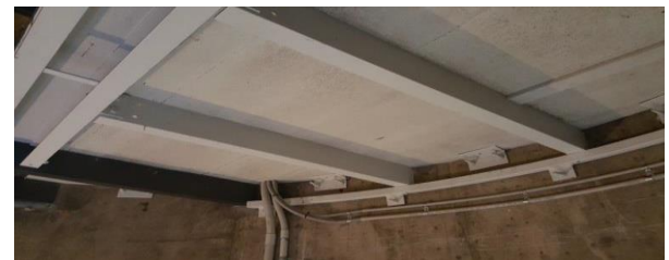
Photograph No. 7B. showing a carrier's air-conditioning cables (related to Photograph 7A) within the water supply reservoir at RFNSA Site No. 4161001 at Alexandra Hills Reservoir located at 36A Alexandra Circuit, Alexandra Hills Queensland.
