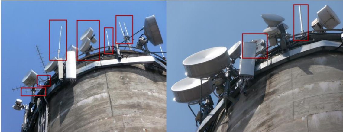
Photographs No. 1 and 2 showing unidentified telecommunication facilities (boxed in red outline) at RFNSA Site No. 4161001 located at Alexandra Hills Reservoir located at 36A Alexandra Circuit, Alexandra Hills Queensland.
