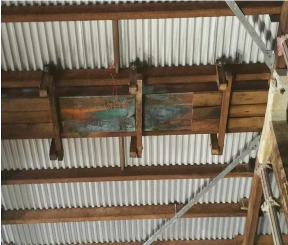
Photograph No. 4 showing roof timber trusses of the reservoir at RFNSA Site No. 4211019 located at Molendinar Water Treatment Plant at Jacobs Road, Molendinar, Queensland.
