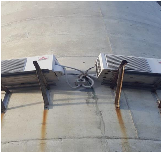
Photograph No. 7A showing a carrier's air-conditioning units attached to the exterior of the water supply reservoir at RFNSA Site No. 4161001 at Alexandra Hills Reservoir located at 36A Alexandra Circuit, Alexandra Hills Queensland. The photograph also shows core cables have been core drilled through the wall of the reservoir.
