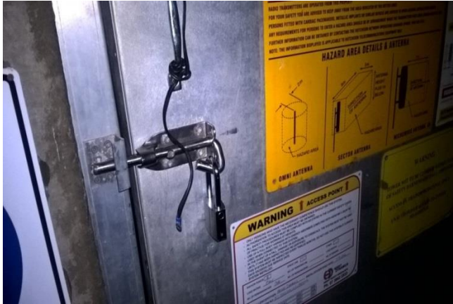
Photograph No. 8 showing lock not installed correctly by a carrier and door able to be opened at RFNSA Site No. 4161001 located at Alexandra Hills Reservoir located at 36A Alexandra Circuit, Alexandra Hills Queensland.
