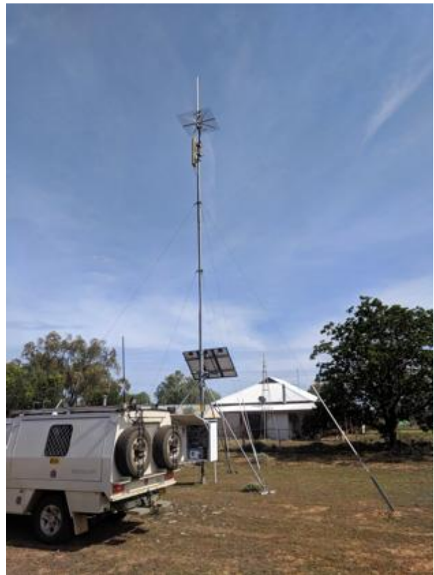
Figure 3 - RMOE Deployed by Telstra
