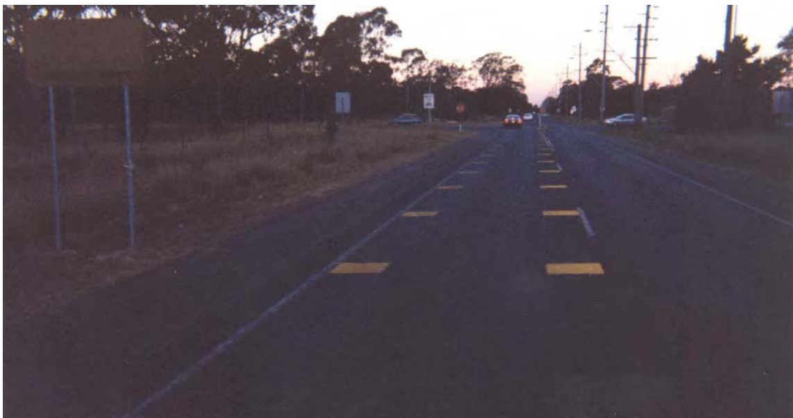
Figure 28: The Driftway at Londonberry Road, NSW: Treatment Site – After Installation of Treatment
