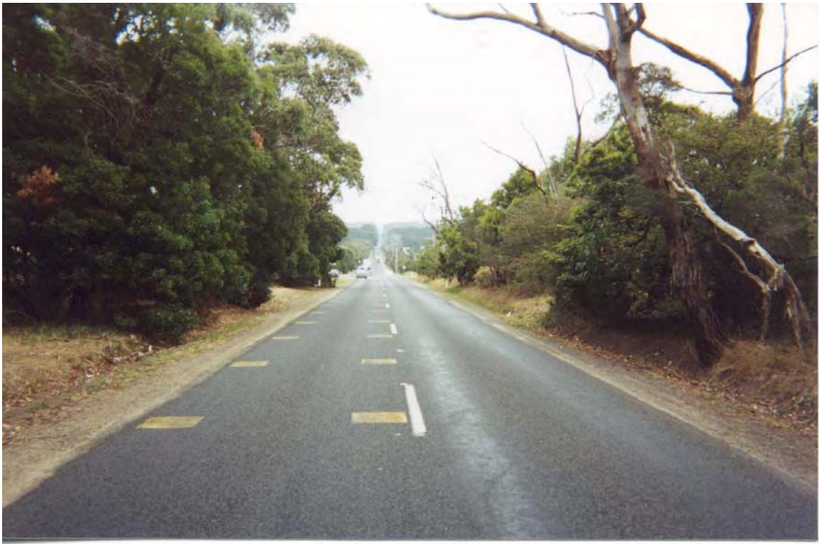
Figure 23: Bittern Dromana Road at Balnarring Road, Victoria: Treatment Site – After Installation of Treatment
