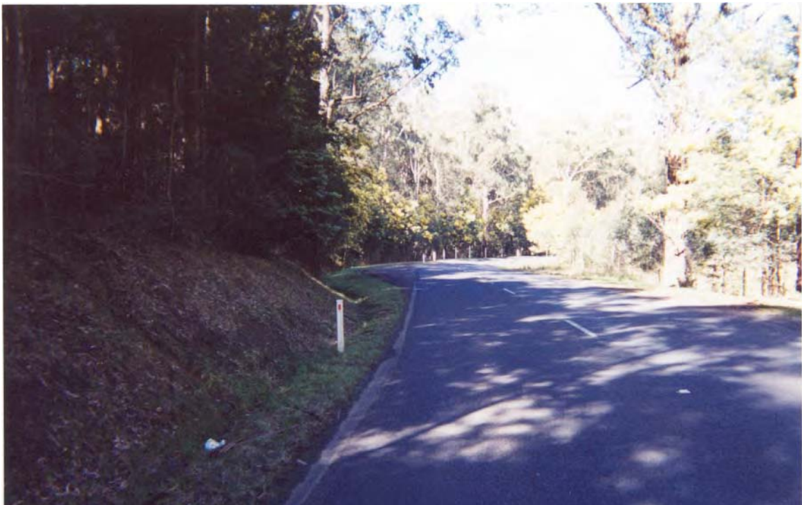
Figure 6: Pakenham Road, Victoria (southbound, north of Mann Road): Treatment Site – After Installation of Treatment
