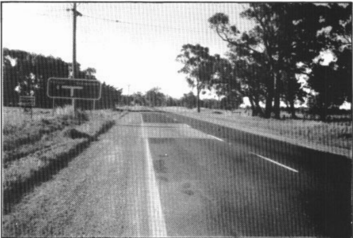
FIGURE 7.2 — Transverse line treatment using different road metal on the Northern Hwy., Victoria.
