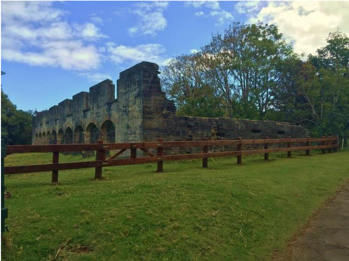
Figure 11: View of safety barrier at the Arched Building, Longridge, 2019. Photo: Australian Government, 2019
