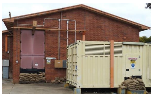
Figure 15: Mudgee Exchange NSW, sandbagged following Burrundong dam spill, October 2022
