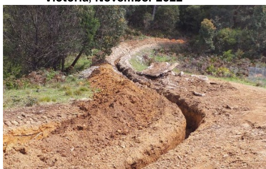
Figure 17: Trenching for a fibre relocation after a land slip threatened a major transmission cable, Falls Creek Victoria, November 2022
