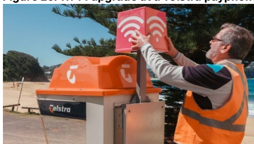
Figure 20: Wi-Fi upgrade at a Telstra payphone
