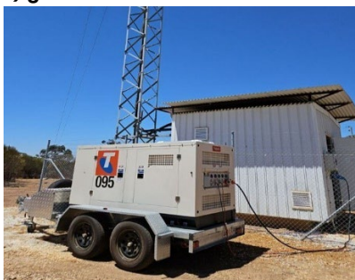
Figure 12: Trailer mounted (portable) generator connected to a mobile hut, Korrelocking, WA, January 2024
