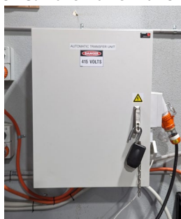
Figure 13: Automatic Transfer Unit
