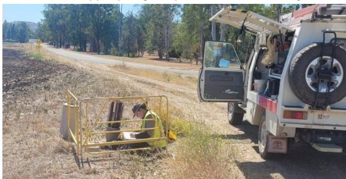
Figure 10: Locating faults on a 56 km copper pair gain system (Australia's longest), Biloela, Qld, Oct 2023
