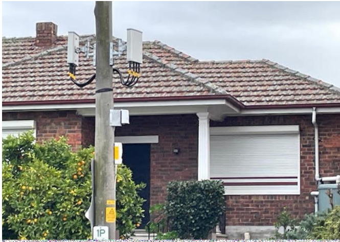
Photo 3: Recently installed Optus pole mounted base station, inappropriately sited too close to a residence
