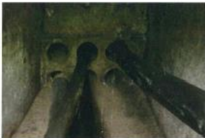
Photo 7- Manhole 'B' looking north across RTA bridge (manhole 'B' to be bypassed)
