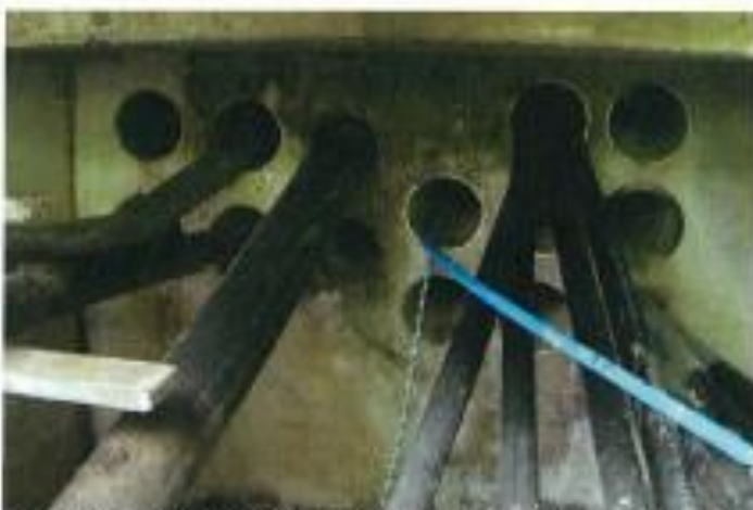
Photo 6 - Manhole 'A' looking south across bridge - 8 way nest of ducts with new cable to be hauled through Duct which already contains blue optic fibre cable
