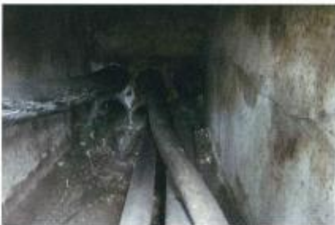
Photo 8 - Manhole 'B' looking south towards Pitwater Road, Narrabeen (manhole 'B' to be bypassed)
