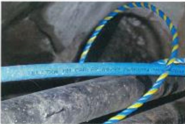
Photo 2 - Telstra optical fibre cable and copper inter-exchange cable located within the Narrabeen duct.
