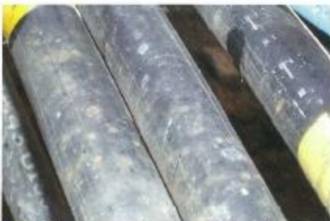
Photo 3 - Large copper inter-exchange cables within the Narrabeen duct.
