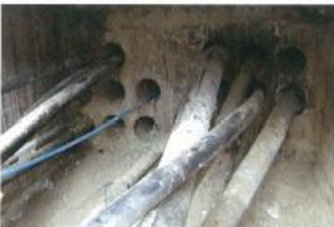
Photo 9 - Manhole 'C' looking north towards the Bridge –8 way nest of ducts with new cable to be hauled through Duct which already contains blue optic fibre cable
