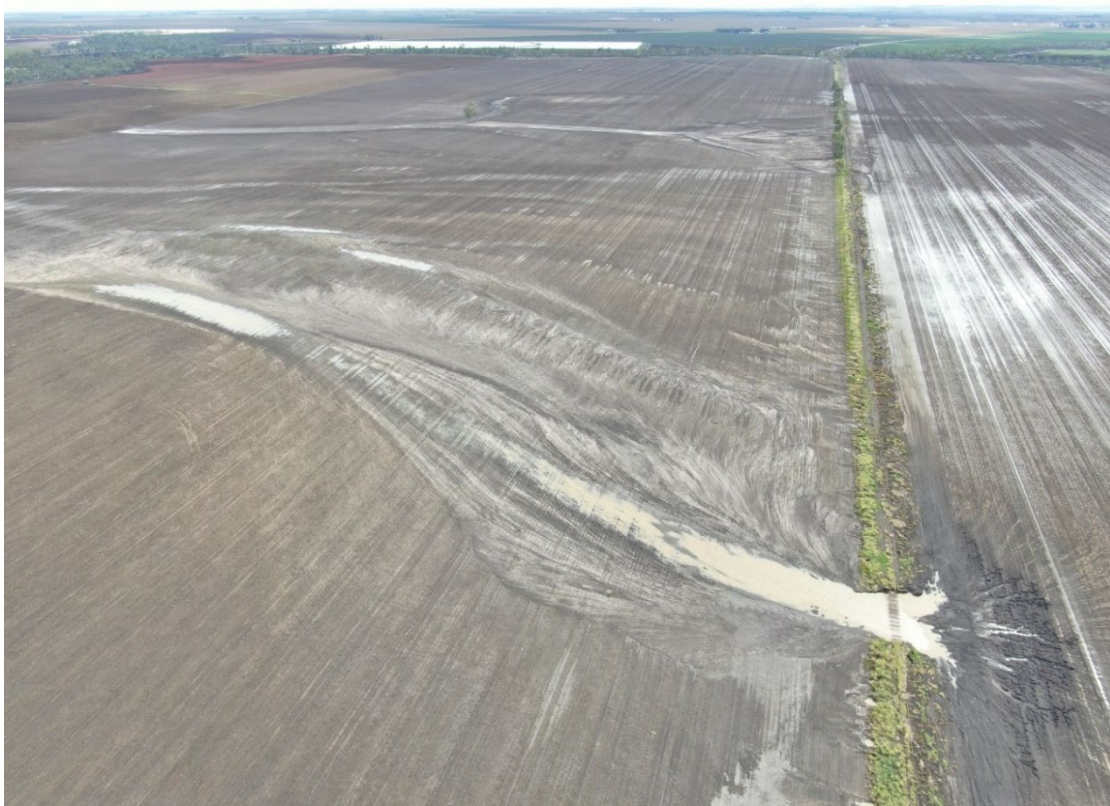
Figure 2: Scour in, and downstream of, the failed culvert, and visible erosion of land adjoining the upstream side of the culvert in the drawdown area.
