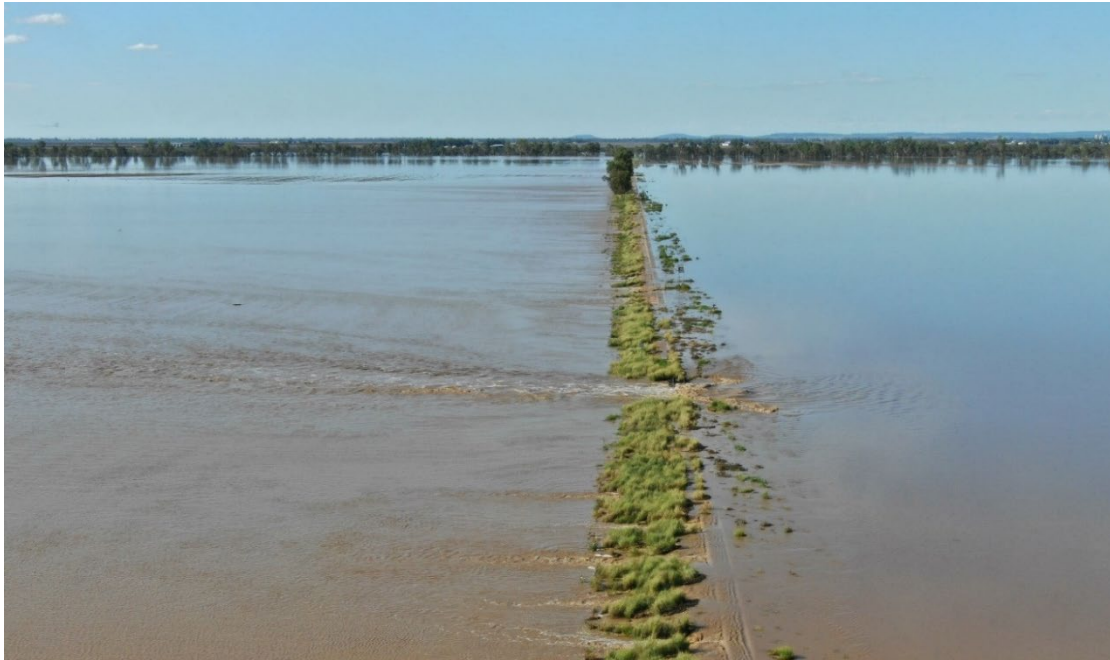
Figure 1: Flood flow passing through a failed culvert in old rail line (property of B. Kelly, Pampas). Flow direction right to left.
