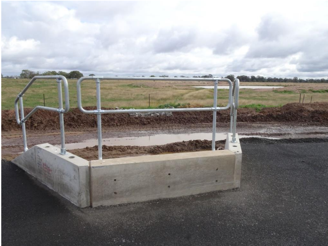
P2N Examples of Earth Mounds Altering and Impeding Floodplains Flow Routing
