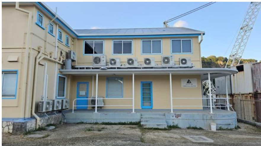
Image: CI Administration building after completion of concrete repairs, corrosion treatment and waterproofing
