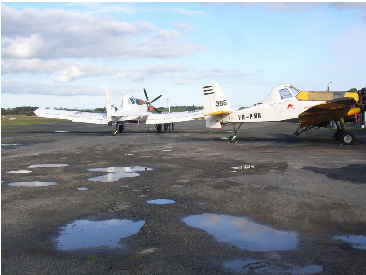
Water ponding on Main Apron after rain
