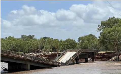
Figure 2: Rapid floodwaters badly damaged the Fitzroy River bridge (approximately 165 kilometres east of Broome, Western Australia) 8
