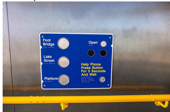
Lift car with help phone linked to hearing loop, Yeronga Railway Station, Brisbane.
