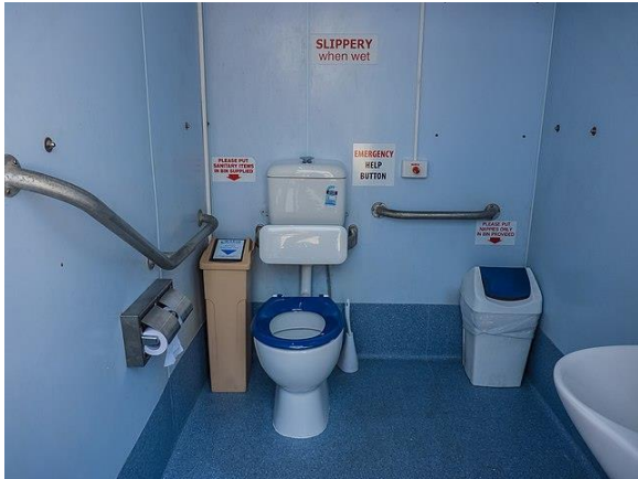
Ferry emergency call button on the rear wall and not reachable from the pan.
