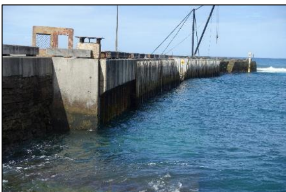
Figure 1-18 View of the western side of Kingston Pier from the boat ramp (Source: Advisian 2020).
