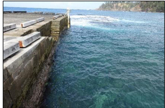
Figure 1-15 View of the southern extent of the western side of Kingston Pier (Source: Advisian 2020).
