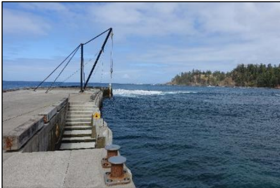
Figure 1-14 View about halfway along the western side of Kingston Pier and the fisherman's crane (Source: Advisian 2020).
