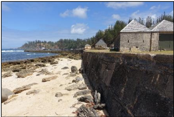
Figure 1-10 View looking west from the foreshore to the Boatsheds and Kingston Pier (Source: Advisian 2020).
