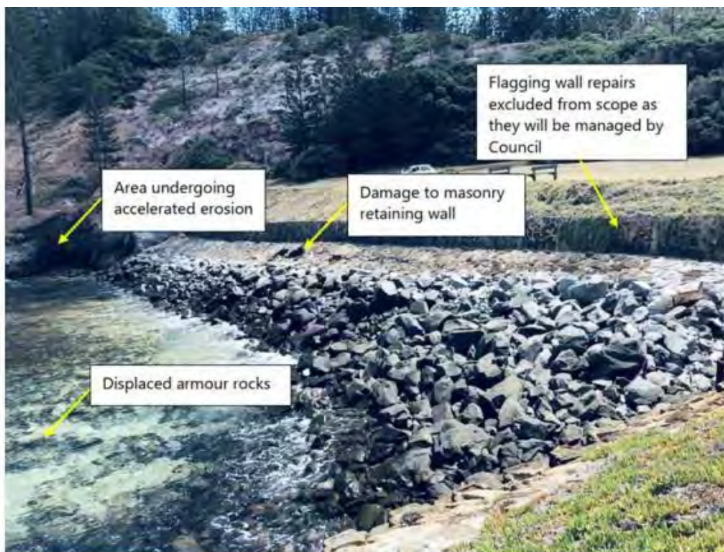
Figure 1-2 Location of rock revetment defects.
